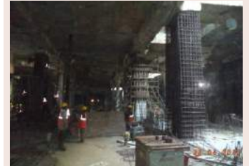
Upper track Plunge in Columns Encasing work in Progress at Central Metro
