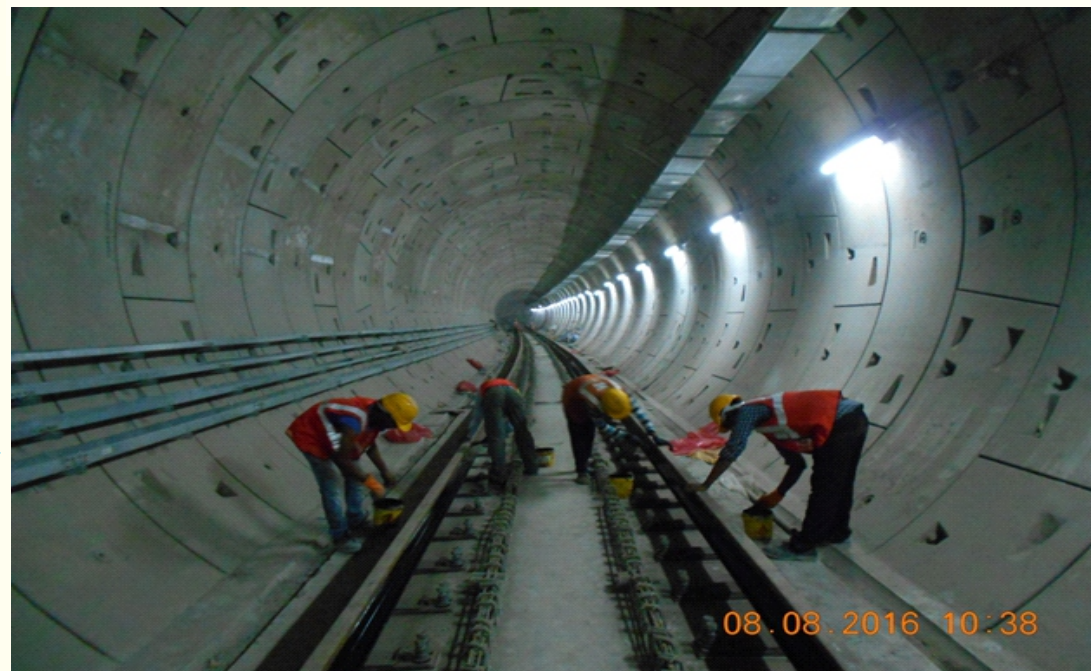
Track Finishing work in progress between Kilpauk Metro and Nehru Park Station
