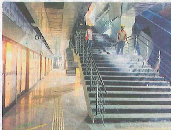
Final touches: Work on the Metro Rail Egmore station is nearing completion. *SPECIAL ARRANGEMENT
