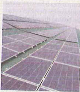
The solar panels on the roof of Alandur Metro stations
